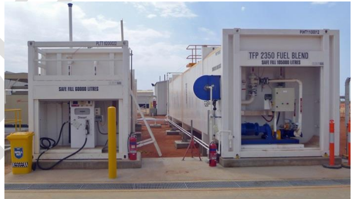
Figure 15. Bulk diesel and fuel blend storage
