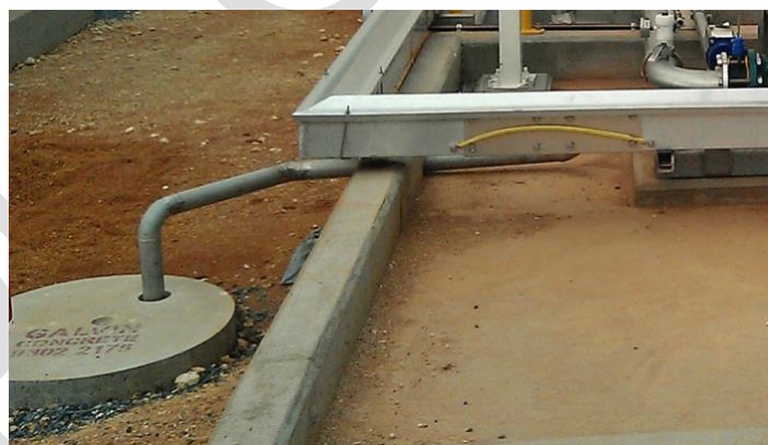
Figure 9. Concrete soak tank
