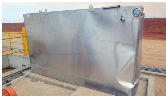
Figure 7. Oily water tank
